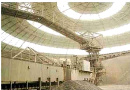
Fig. 10. Stacker and Reclaimer
